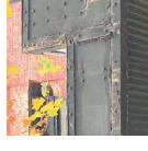
SF Steel fascia Restored + reconstructed to match exist Paint finish - protective coating Colour: Bronze to 191-195, Dark green to 197-199+201 Location: Street awning fascia
