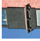
TP-E Painted timber - existing Repaired with new paint finish Location: Existing timber cladding & trim
