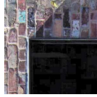
SW Steel framed window Clear glass Location: Windows to fire stair (sprinklered)
